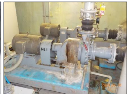
cooling water pumps for air conditioning in the main building
