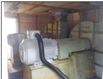
scrubber exhaust fans
