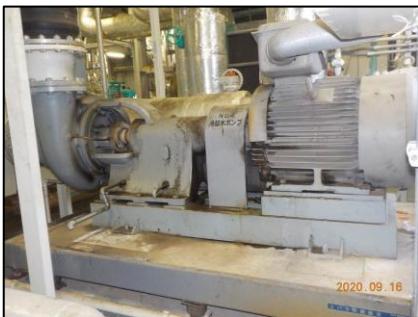
cooling water pumps for absorption refrigerators
